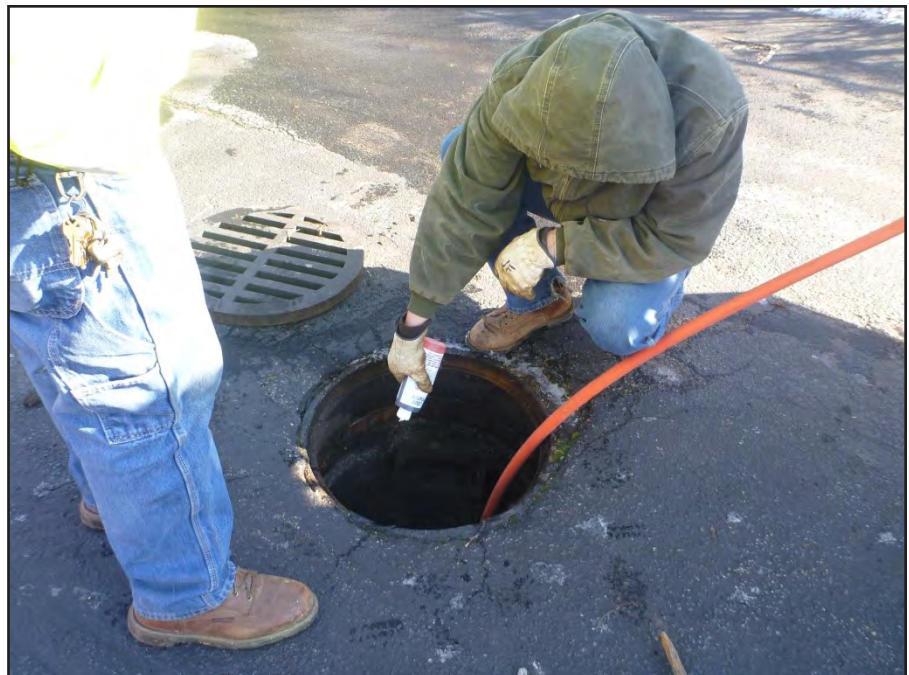
Figure 7. Dye tracing being conducted in the city sewers of Somerset.
